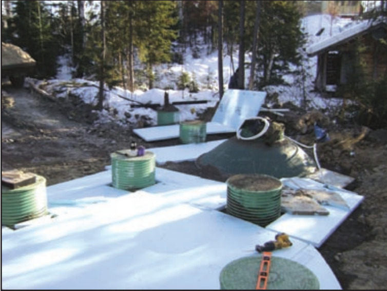
Insulating tanks at a Northern MN Camp
