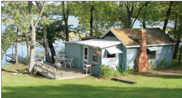
Rugged River Resort's Cabin 4 had a 100+ years of history, been patched again and again and was in need of replacement.
