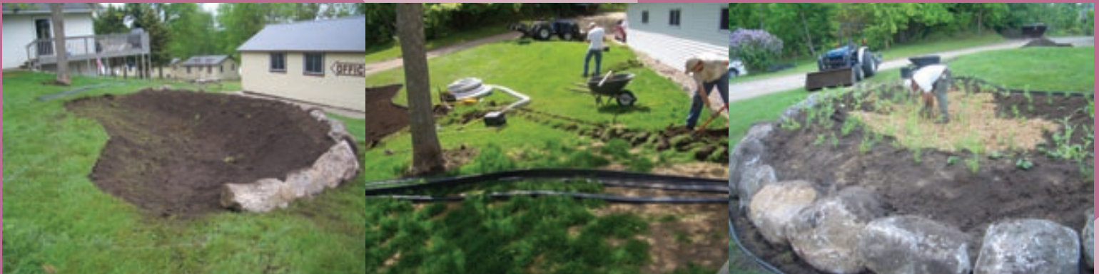
The Prosofskis designed and constructed a rain garden on their resort to curb the negative impact of water runoff. Above are a series of photographs marking the construction progression of the rain garden.
