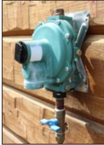
At the cabin, you should have a secondary regulator that changes the pressure from about 10 psi to 11 – 13 inches of water column.
